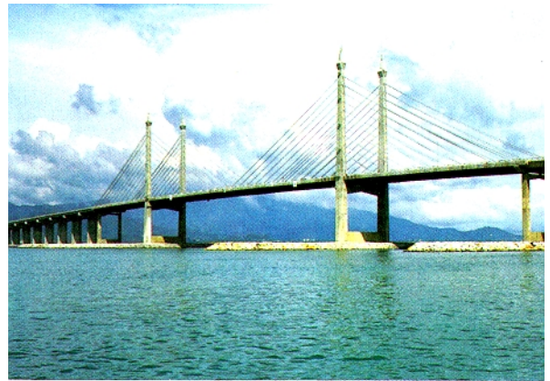
This cable-stayed bridge, designed by HNTB, has a main span of 738 feet. It was opened in September 1985.
