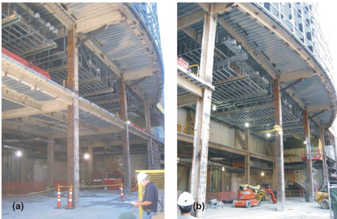
Figure 7. Lobby Renovation, 100 High Street, Boston, Massachusetts. (a) Before: columns and cantilevered girders reinforced prior to removal of three 30 ft x 30 ft bays. (b) After: three bays of slab framing removed, and column reinforcement completed.
